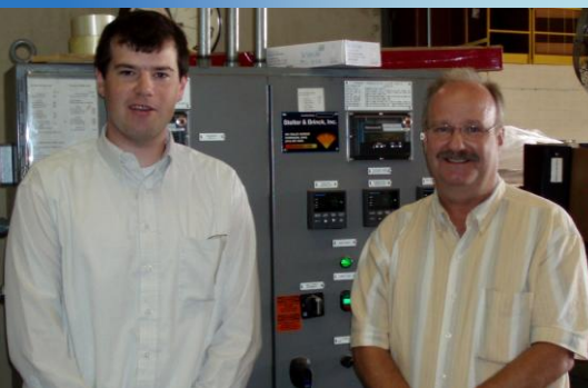
Tony Brinck from Stelter & Brinck and Randy Corns from 3-Sigma in front of a Stelter & Brinck control panel.
