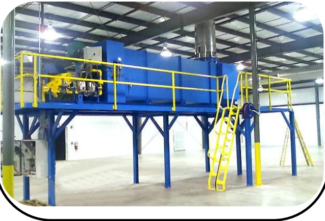
Below: S&B oxidizer installed at Bontex.
